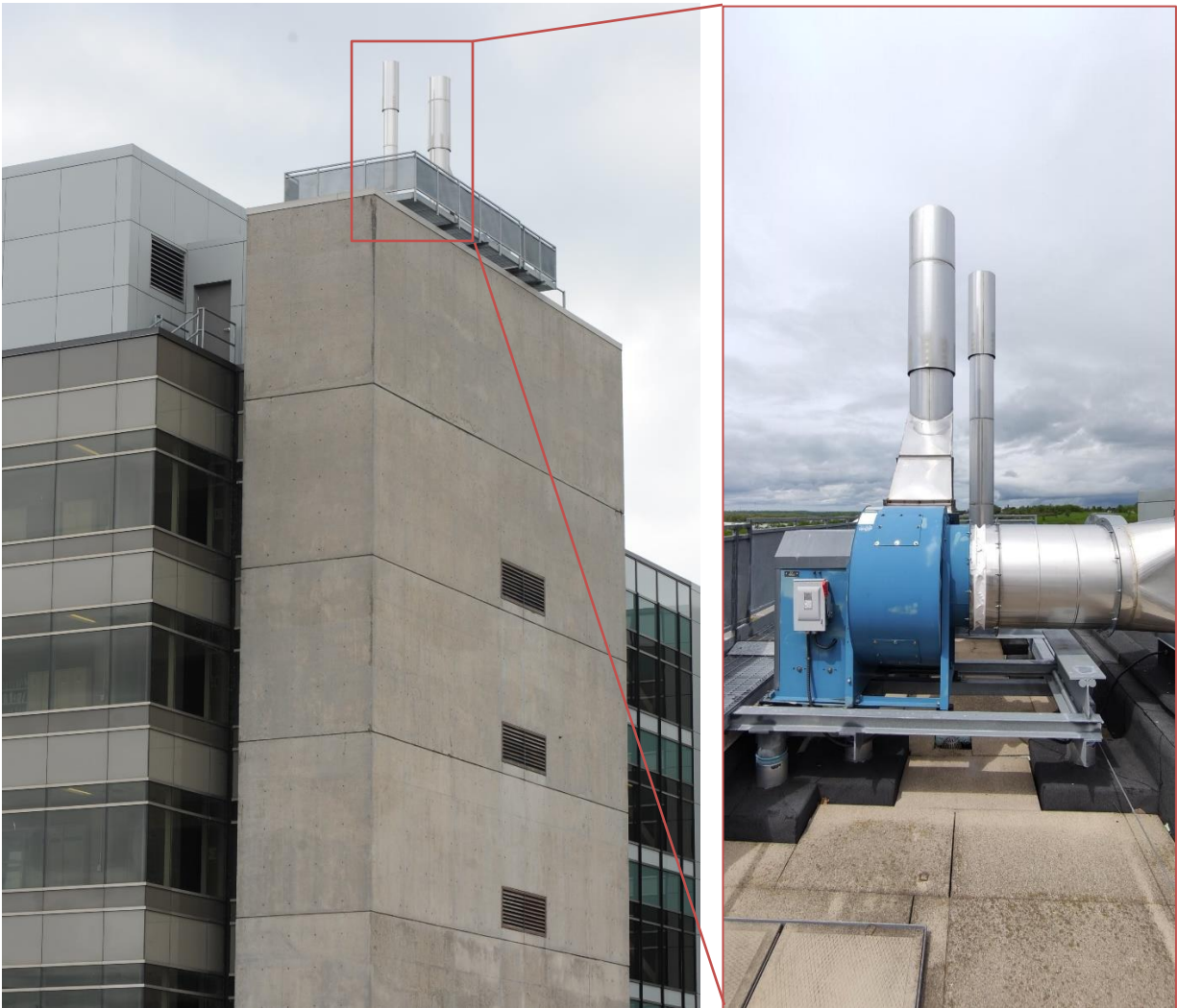
Figure 4. Left: West side of the Sawyer Engineering Building Module 5 with visible exhaust stacks on the roof highlighted in red rectangle. Right: Exhaust fan motor (blue) and exhaust stacks for the SLOWPOKE-2 Facility at RMC on the roof of Sawyer Building Module 5.
